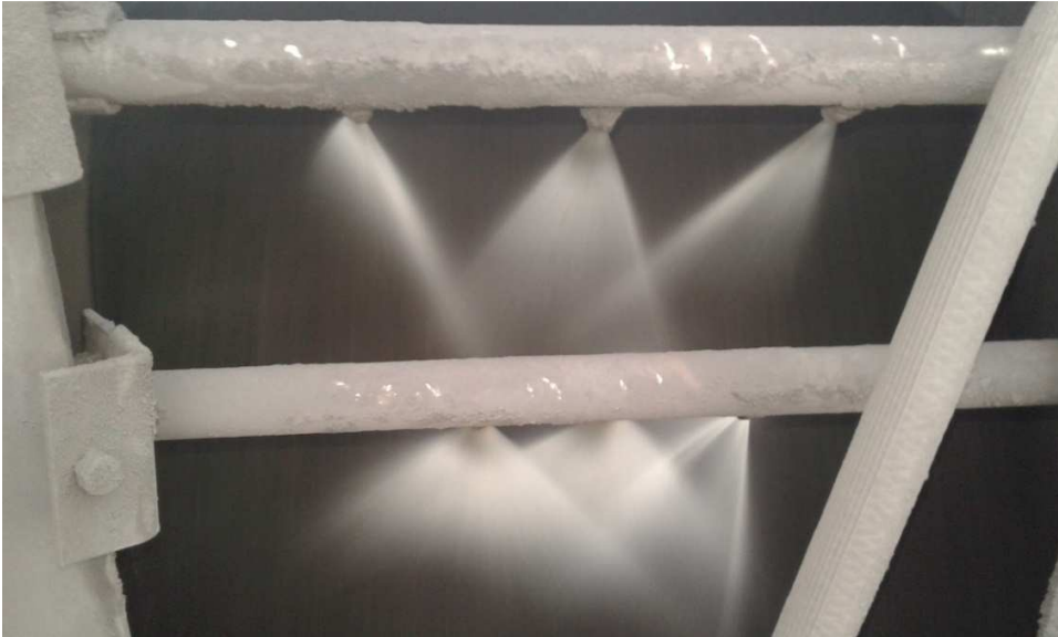
Figure 7.1. Treatment Manifolds at UMK
