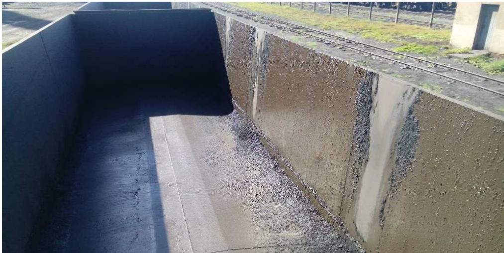
Figure 7.6. Residual material due to rainfall
